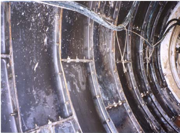
Figure 2. Damage to liner plates in one tunneling application at an estimated jacking load of 240 tons.
