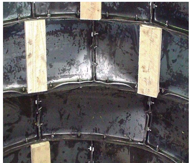
Figure 14. Timber planking transfer loading and cause damage to the flange area below with no apparent damage to the timber planking.
