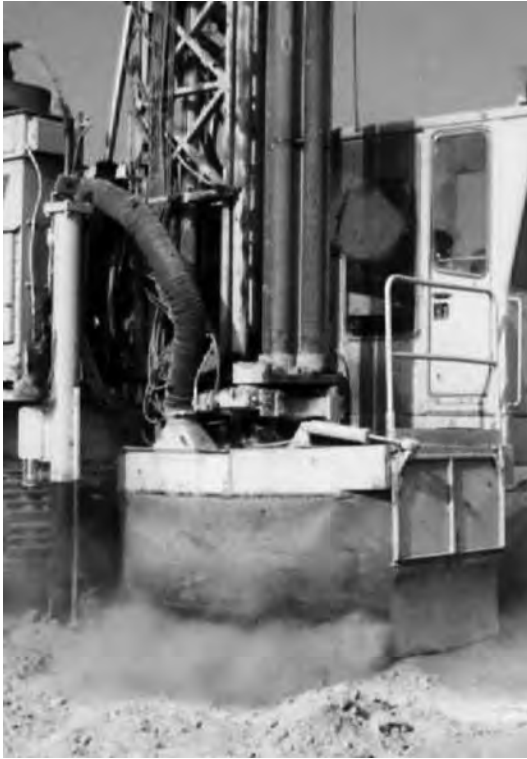
Figure 1 — Drill deck with shroud showing leakage between the bottom of the shroud and ground surface.
