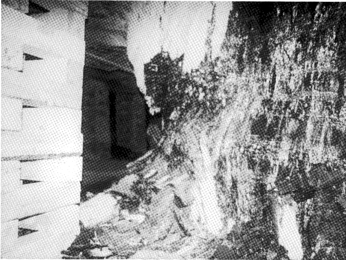
Figure 4.—Rib experiencing brittle and slabbing failure.
