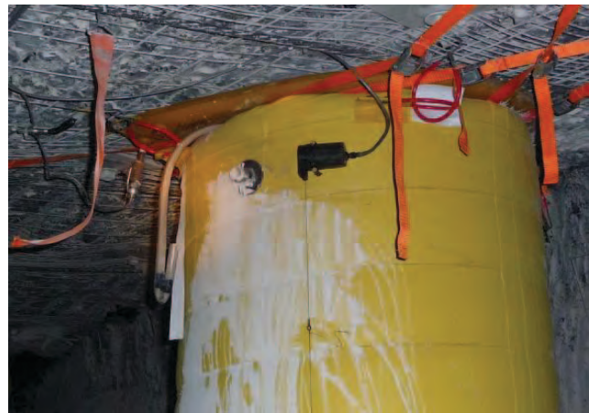
Figure 5. Load cell and displacement transducer installed on a pumpable crib.
