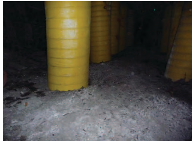
Figure 12. Floor heave developed during first panel mining from the side abutment at Mine B.
