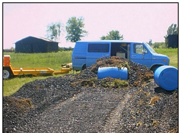
Figure 6.—First layer of coal covering electrode grid and first perforated plastic barrel being covered horizontally on coal pile.
