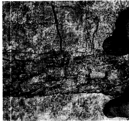
Figure 4. Disrupted zone of closely spaced mining-induced extension fractures indicating activation of zone as a flat fault.
