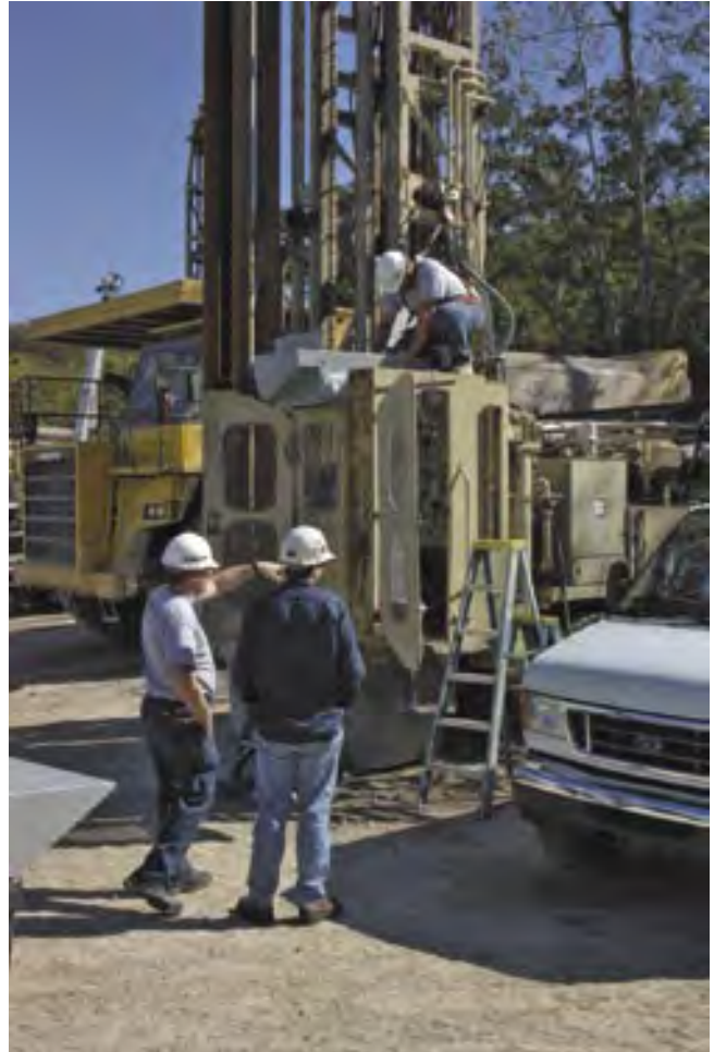
These drill operators are busy installing a new unidirectional filtration and pressurization system.
