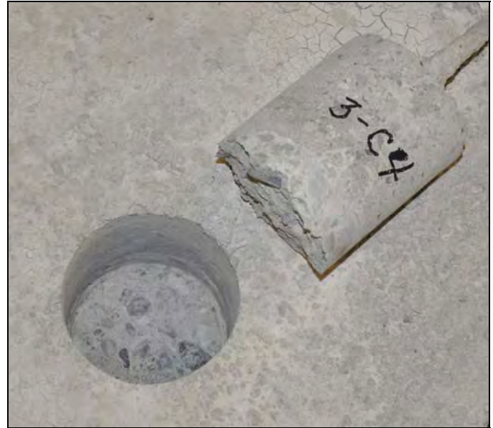
Figure 16. Adhesion test specimen showing a tensile failure surface located predominantly in the concrete substrate.
