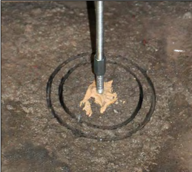
Figure 15. Parallel and concentric drill holes with extension rod connected to epoxied stud.
