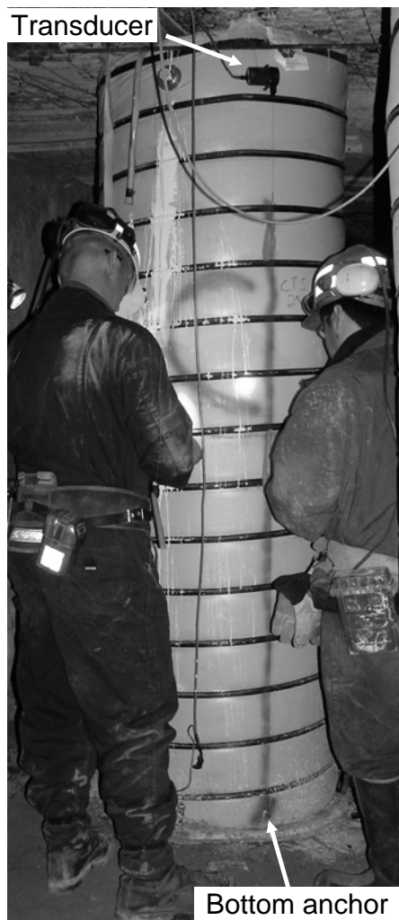
Figure 3. Convergence instrumentation shown on pumpable roof support in longwall tailgate.
