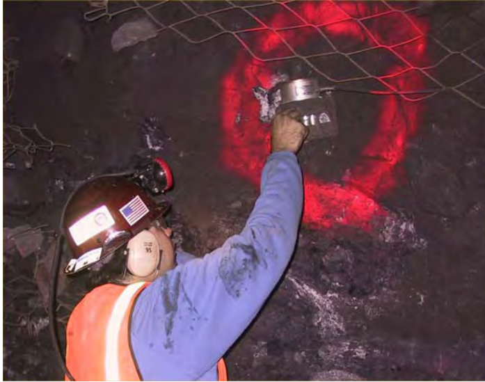
Figure 3. Installing a triaxial transducer and bracket on the rib in XC 11.
