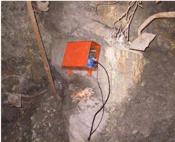
Figure 4. Seismic monitor C installed in an armored steel box in XC7
