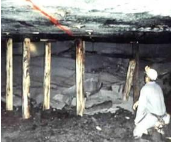
Figure 3. A roof fall, at least 5 ft high, has blocked the entry. The timber supports were installed later.
