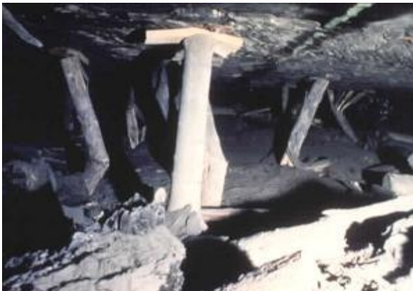
Figure 6. A pillar squeeze has resulted in closure of the mine entry and damage to the supports.
