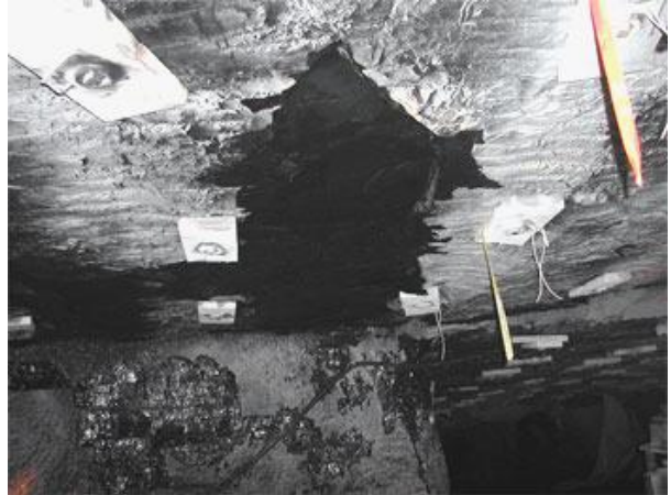
Figure 4. A piece of rock 4 ft wide, 10 ft long and just several inches thick has fallen from between the roof bolts. This rock fall resulted in a fatality.
