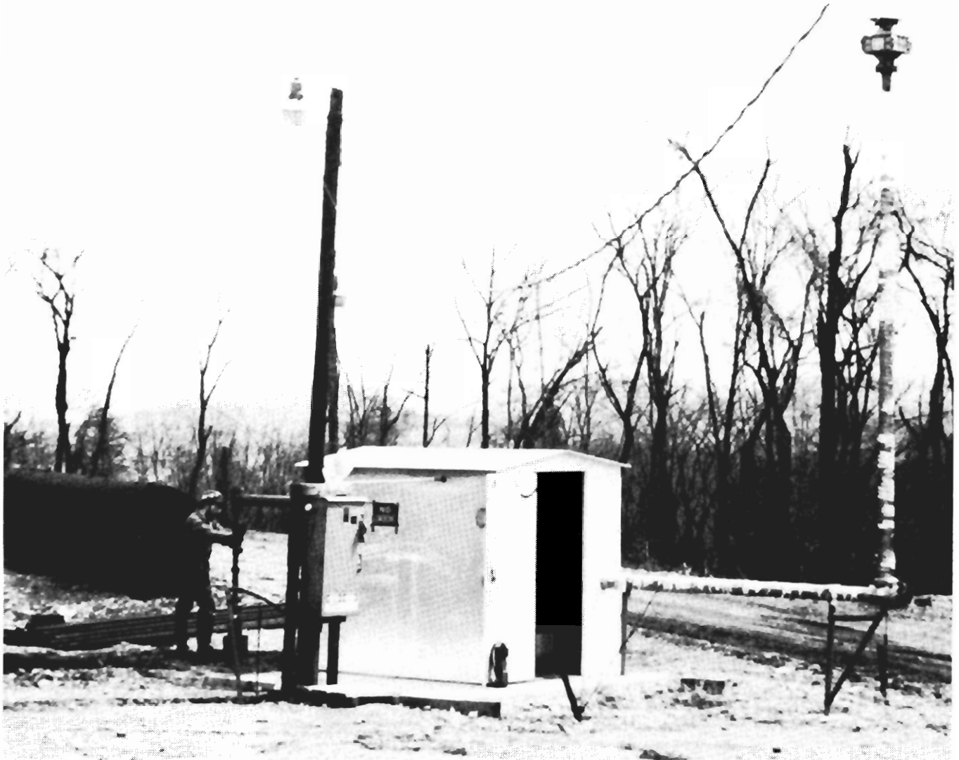
FIGURE 21. - EM-19 surface installation. Wellhead and pump control panel at left.
