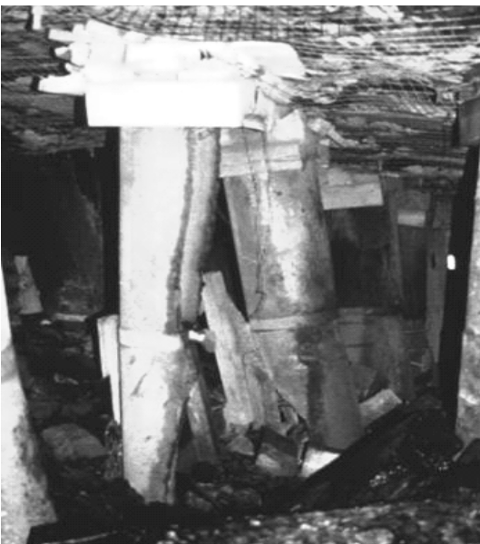
Figure 10 – Failure of high capacity concrete crib in longwall tailgate.
