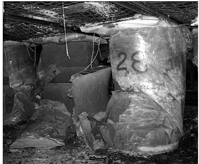
Figure 11 – Failure of high capacity concrete crib in longwall recovery room.
