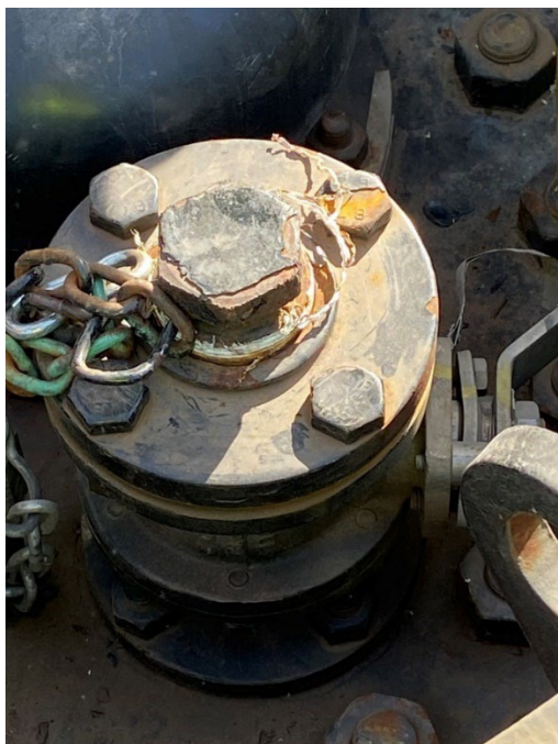
Figure B9. Valve inside the housing with a damaged seal on the valve cover. Photo by NIOSH.
