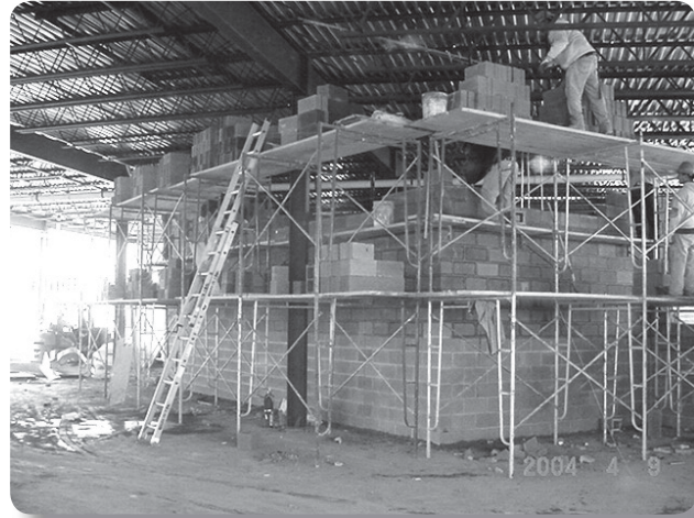
Problem: Conventional unguarded frame scaffolding
