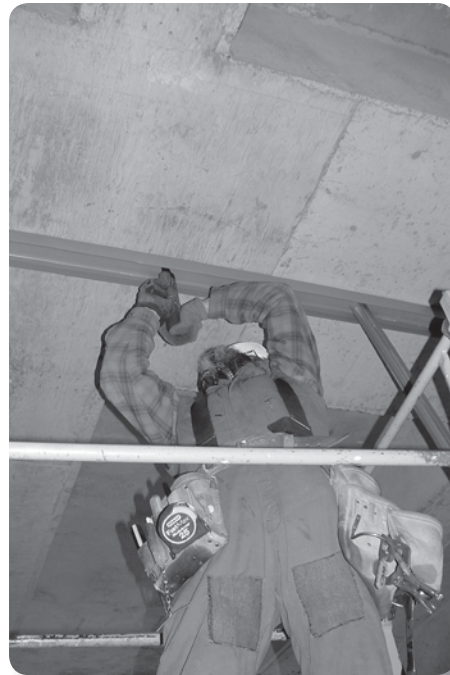
Problem: Using PAT overhead
