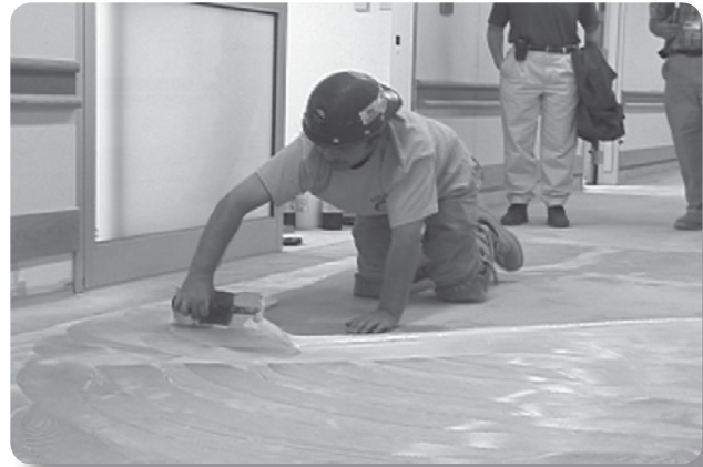
Problem: Kneeling to work near floor
