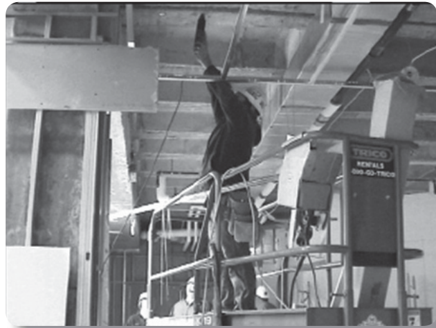
Problem: Drilling overhead
