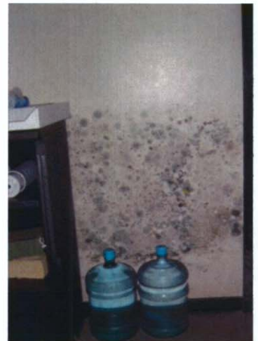
Mold growth on wall board.
