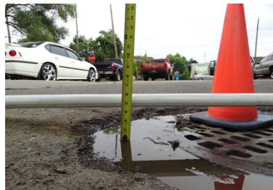
Figure 4. Storm drain cover/pavement condition at incident
