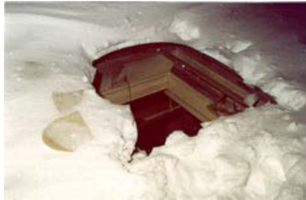
Figure 1. This picture shows the broken skylight where victim fell.
