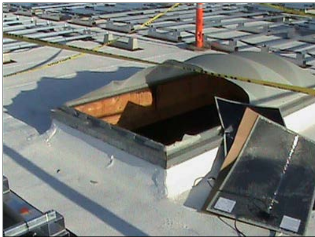
Exhibit 3. The skylight the victim fell through.
