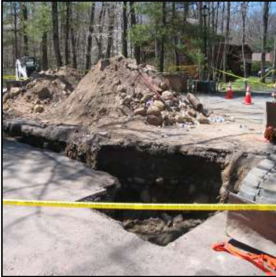
Figure 3: Location of collapse. Note spoils piles and equipment located less than 2 feet from the edge of the trench (courtesy of OSHA)
