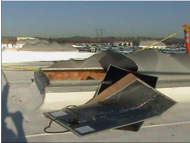
Exhibit 4. The solar panels that the victim was carrying when he tripped.
