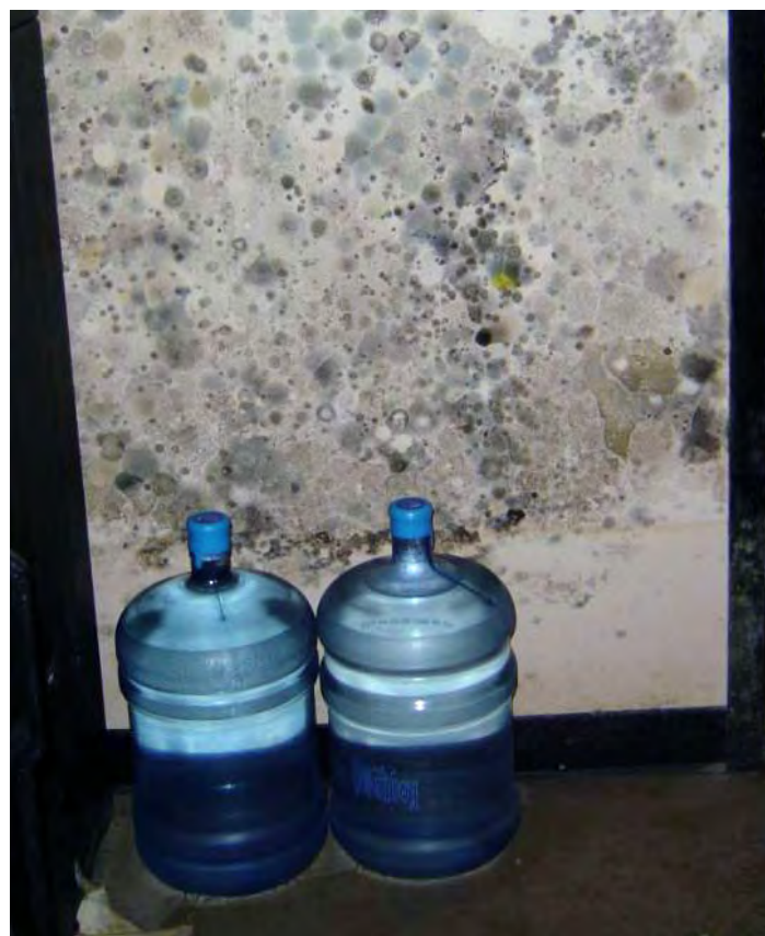
Mold growth on wall board.
