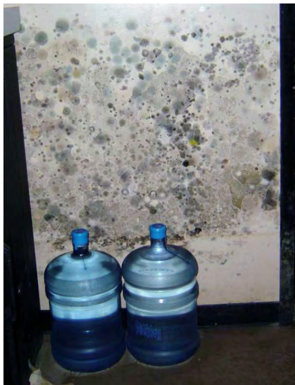
Mold growth on wall board.
