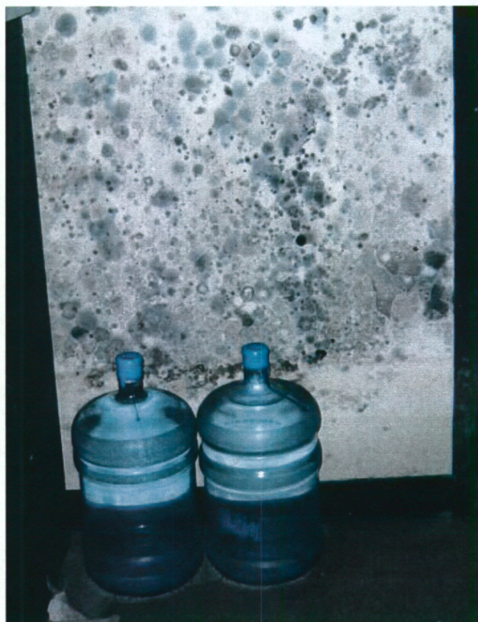
Mold growth on wall board.
