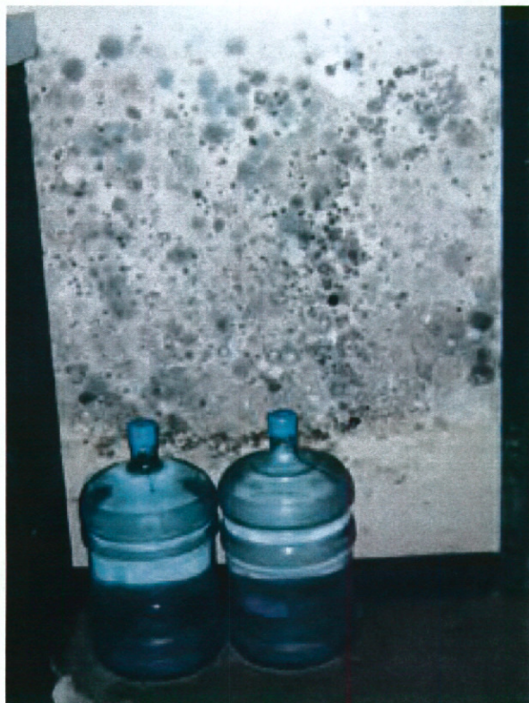
Mold growth on wall board.
